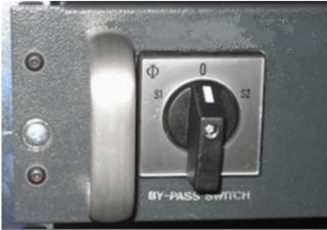
Fig. 11 – Bypass switch QS1
