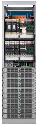
Combination Power and Distribution Bay
