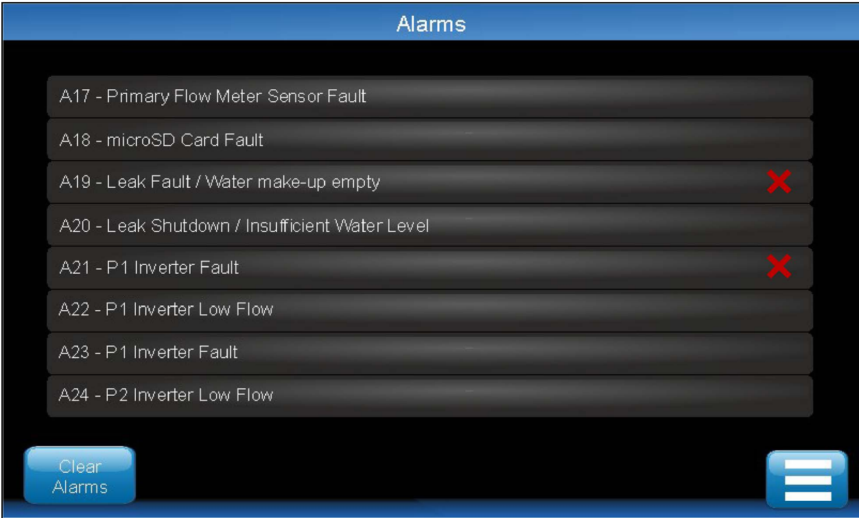
Figure 4.18 Control Screen Alarm Identification
