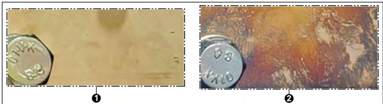
Figure 4.6 Cable Landing Busbars
