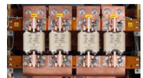
Battery / Load Connection Unit
