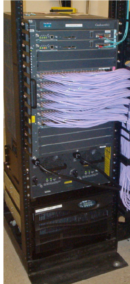
A network closet at Marquette.
