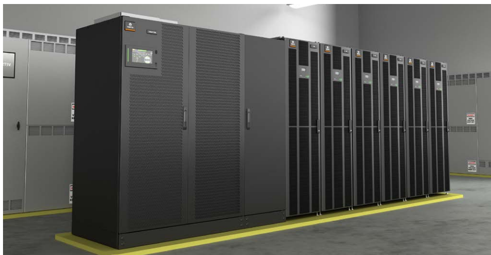
Vertiv™ HPL Lithium-ion Battery Cabinets with 1200kW Liebert® EXL S1 UPS
