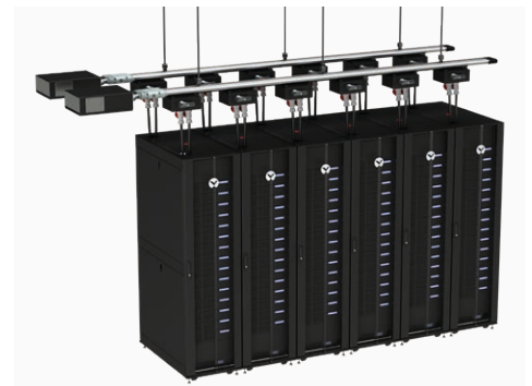
Data Centre with Vertiv™ Powerbar iMPB
