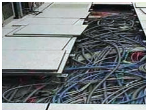
Typical Data Centre with Power Cables and Conduit
