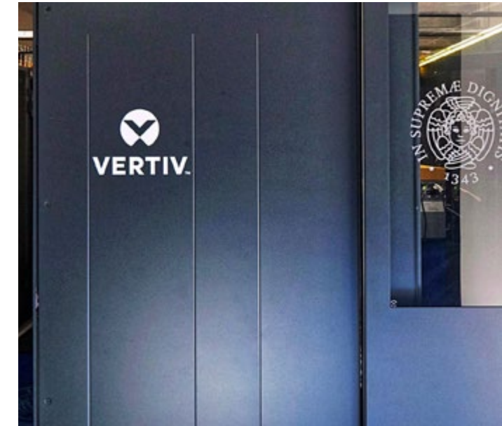
Among the main benefits provided by Vertiv solutions is the implementation of liquid cooling in existing air-cooled data centers.
