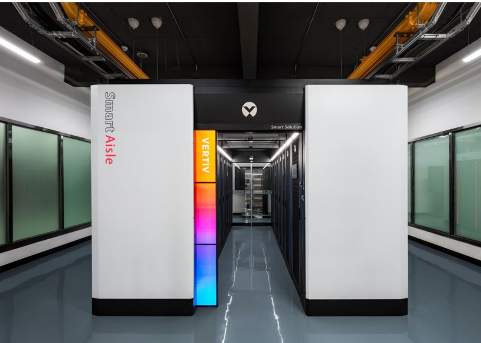
The Vertiv™ SmartAisle™ 3, an AI-enabled micro-modular data center solution, is a centerpiece of the customer experience center and academy Shenzhen, China.
