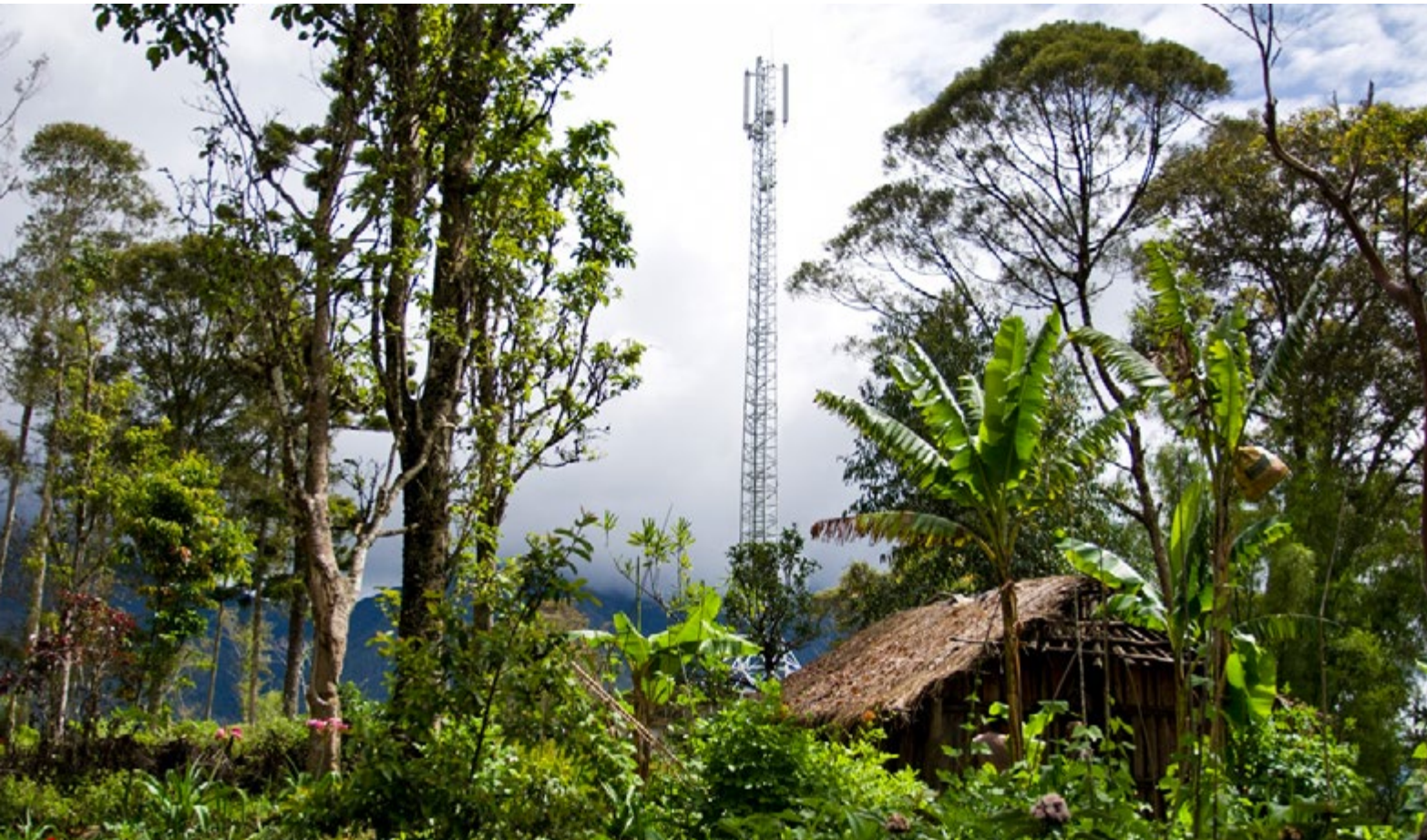
A newly installed system in the mountains of Papua New Guinea enables cell phone coverage through the use of solar energy solutions.
