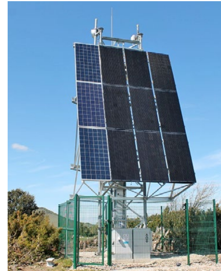
Usage of solar energy provides flexibility to install a repeater in the right location in France.
