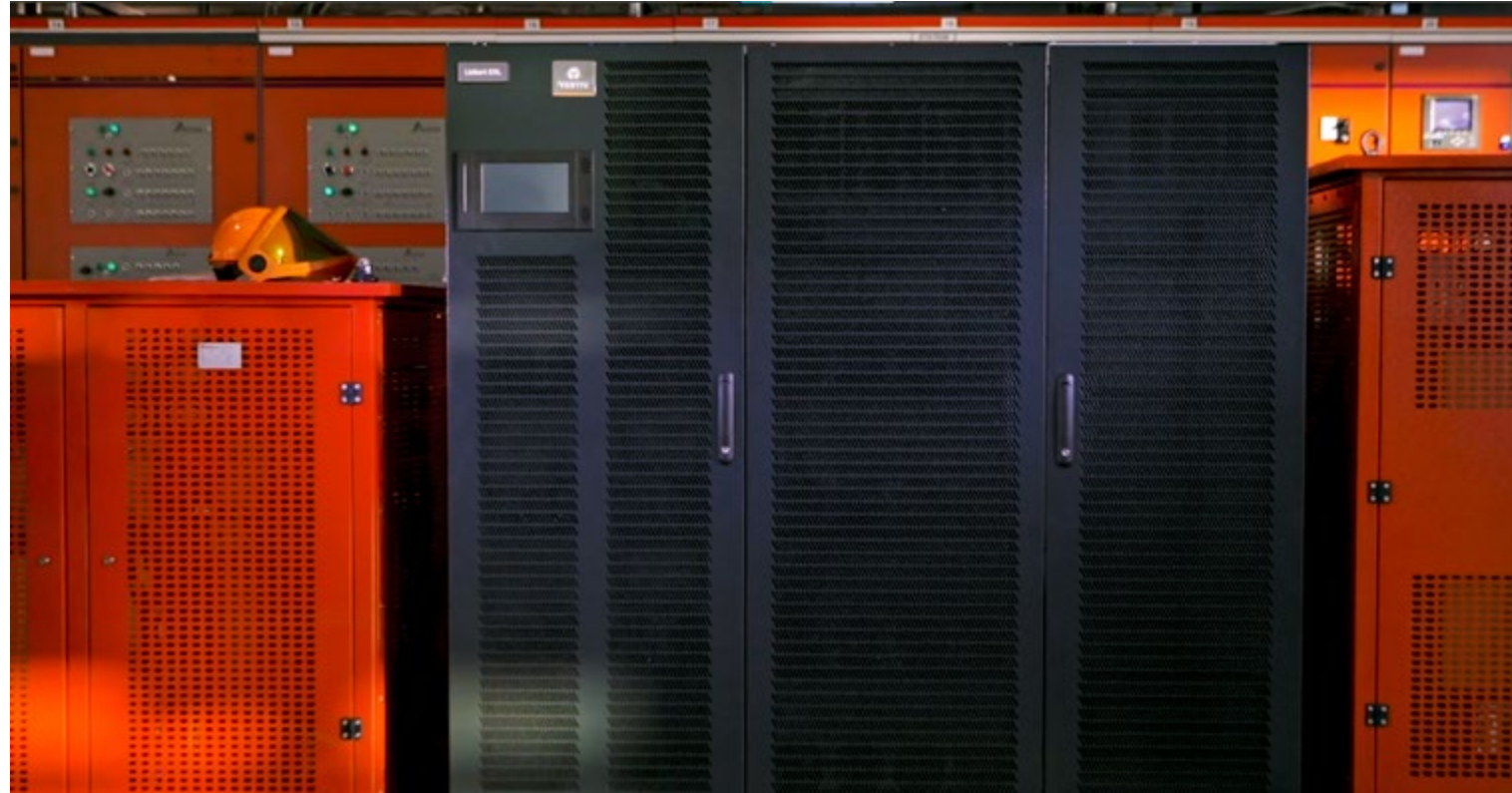
A Vertiv™ Liebert® EXL S1 UPS undergoes factory acceptance testing at the Castel Guelfo customer experience center in Bologna, Italy.
