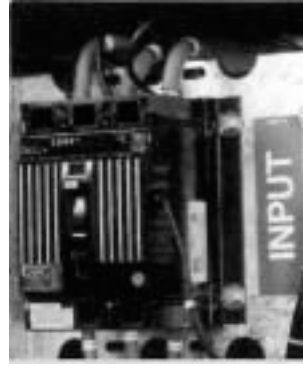
Input circuit breaker
