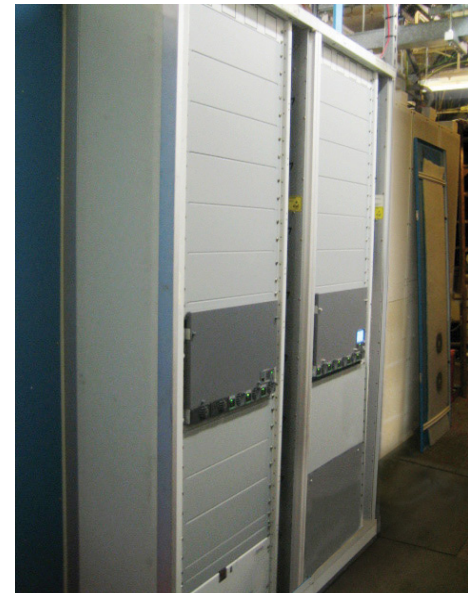
After: Legacy system retrofitted with NetSure 5100
