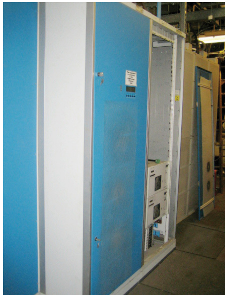
Before: Legacy Ericsson DC Power System
