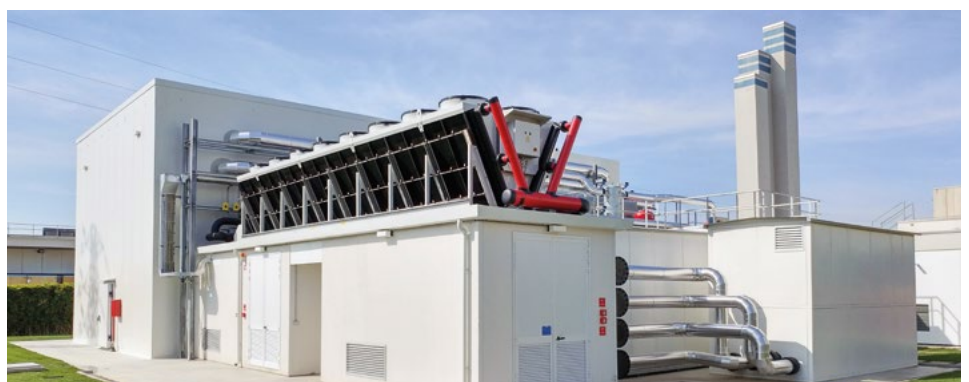
Adiabatic Freecooling Chiller Innovation lab
