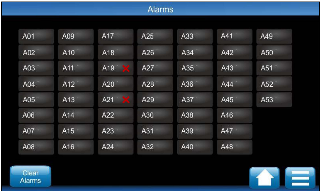
Figure 4.17 Control Screen Active Alarms
