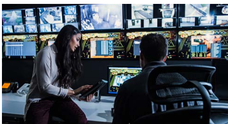
Process Control Rooms
