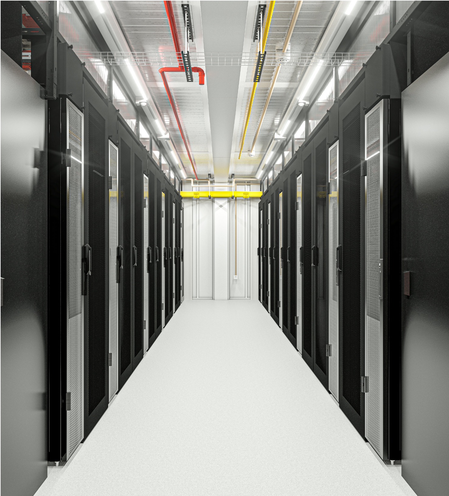
Interior view of SmartMod Max
