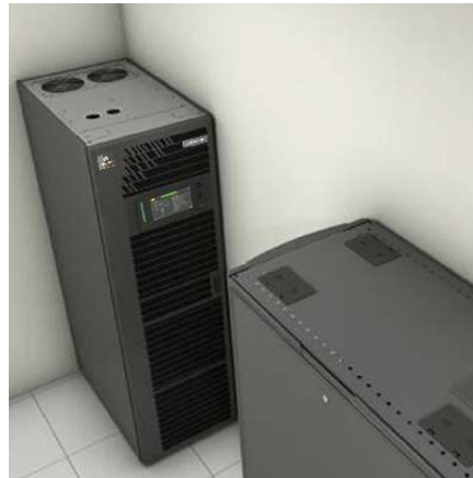
Liebert EXM detached from the wall
