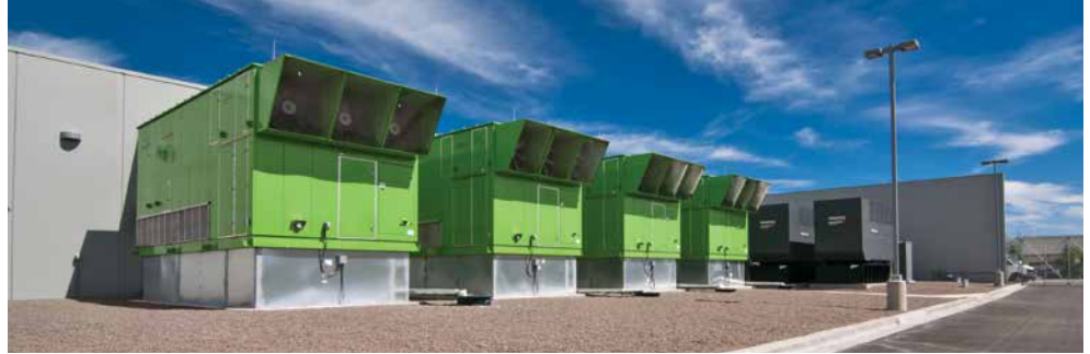
Liebert Indirect Evaporative Freecooling Units deployed at Green House Data, Cheyenne, WY
