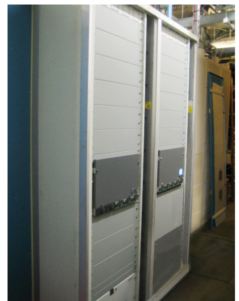
After: Legacy system retrofitted with NetSure 5100
