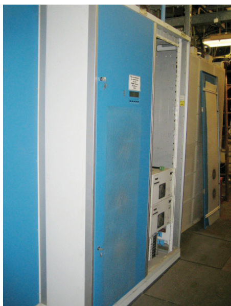
Before: Legacy Ericsson DC Power System
