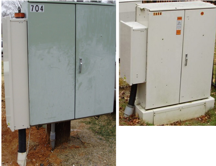
Figure 1: Completed Add-On 400 Pr. Annex NetReach™ Expander® Cabinet Installation (left-hand installation shown for left: 1x8 Expander® cabinet and right: 2x4 Expander® cabinet).
