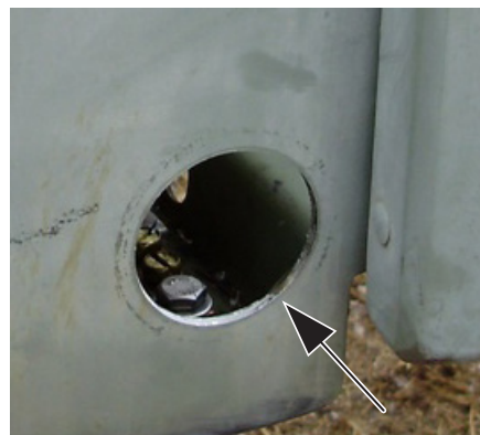
Figure 5: Marked and drilled 1-3/4" hole at the lower left-hand side of the host Cross-Connect cabinet.
